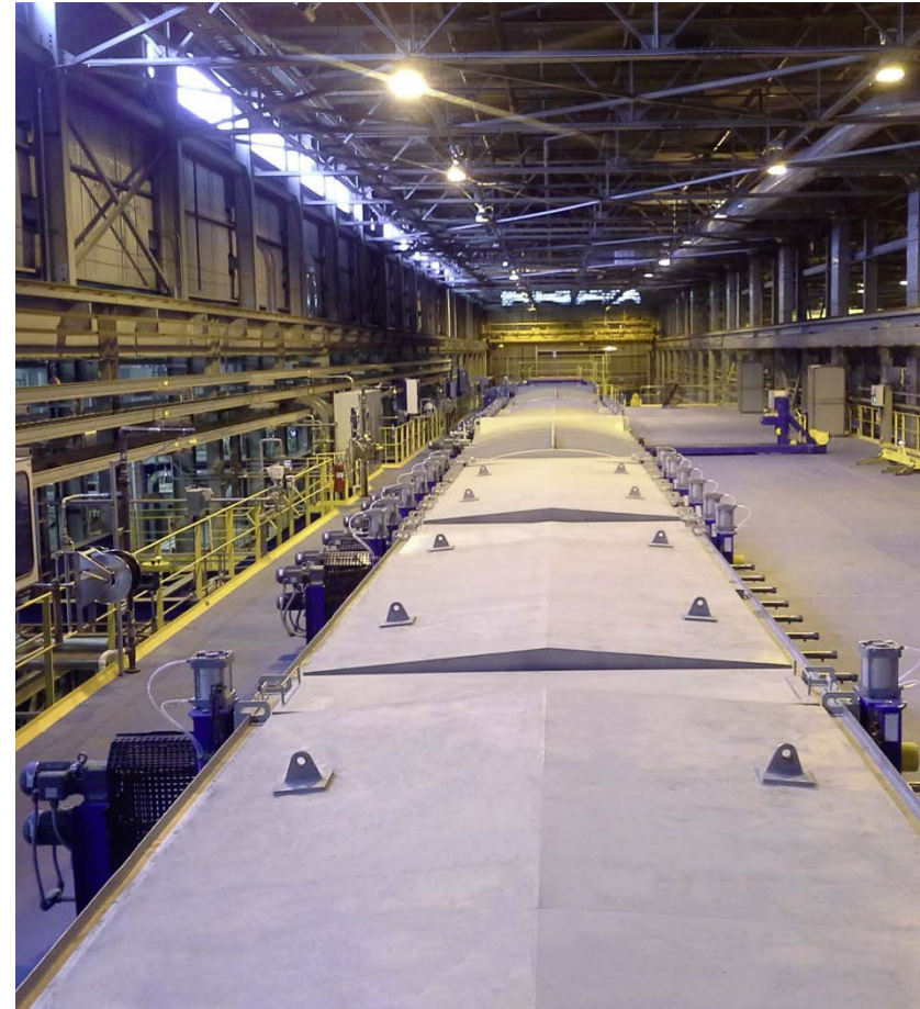
▲ Overview of a chemical treatment line
